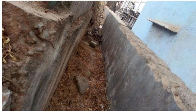
Fig:3.3 Improper drainage system
