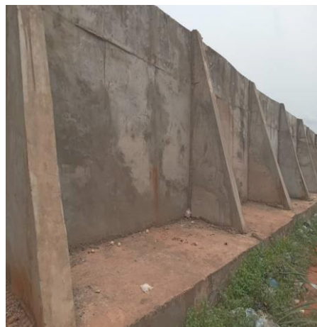
Figure 1: Water Defense Wall
