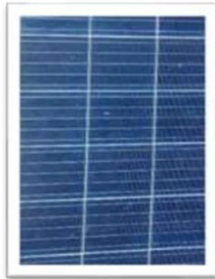
Fig. 05 Solar panel without Dirt
