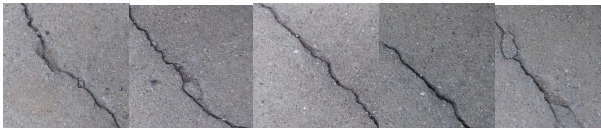
(a) Crack Images
