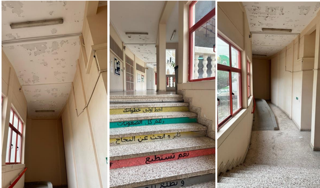
Figure 1. Peeling paint on the ceiling, dust and dirt accumulated on the ground (Source: Author)
