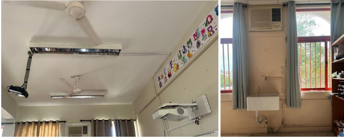
Figure 3. Faulty electrical solutions in the classrooms and exposed water pipes in the art studio (Source: Author)
