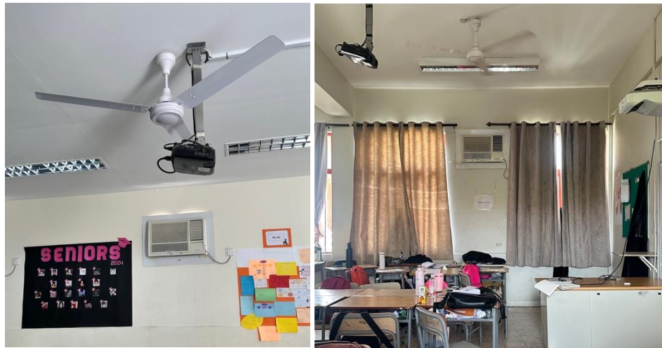
Figure 7. Window air conditioners are the mainly used cooling system (Source: Author)
