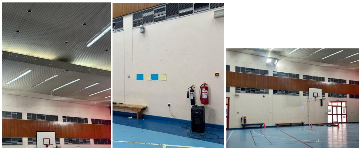
Figure 2. Broken AC grills and non-working lighting, and dirt accumulation on the ground (Source: Author)
