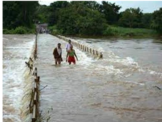
Fig. 1 : A typical bridge flooded with water
